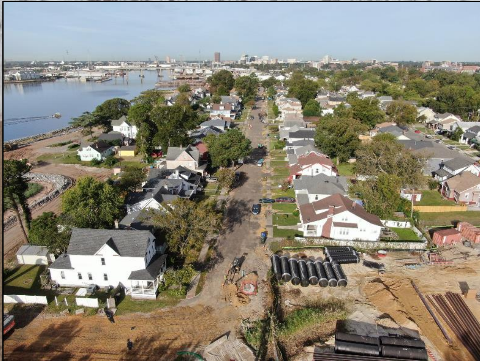
Chesterfield Heights , October, 2020 ~ photo courtesy of MEB General Contractors/ City of Norfolk
